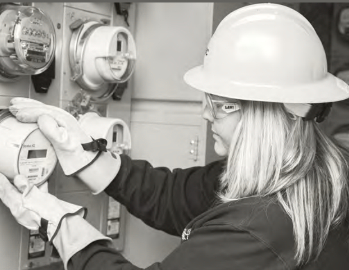
NOVEC Field Services Technician Candace Burns installs an advanced meter at an apartment building in Manassas.
